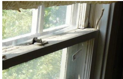
Missing glazing and paint, minor frame rot
